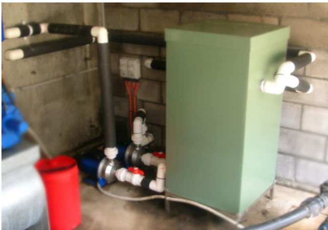
Glycol Storage Tank and Circulation Pumps
